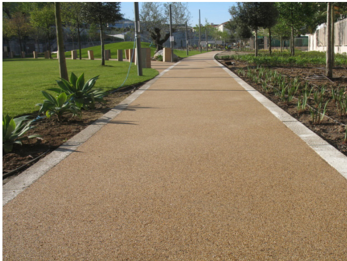
Self binding gravel to access drive plots 6-10, and footway to drive from Ilsham Marine Drive
